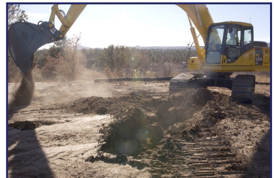
A backhoe lifts the first shovel of dirt for the new Radiological Laboratory Utility Office at TA-55. Photo Credit: LeRoy N. Sanchez, LANL Public Affairs
